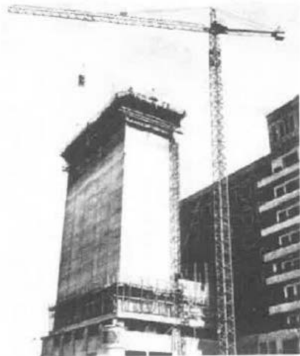
View of the construction of the Silo for the flour industry "MILLS AG, GEORGIJOU"
