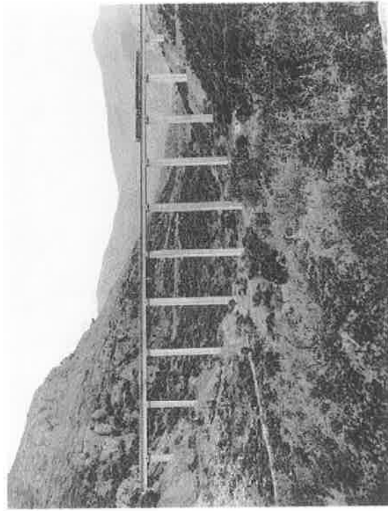
Bridge of Achladokampos (the first rail bridge in Greece made of concrete with pillars of 60m)
