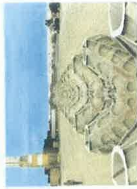
Arrangement of the moulds for the fabrication of blocks of concrete in JUBAIL
